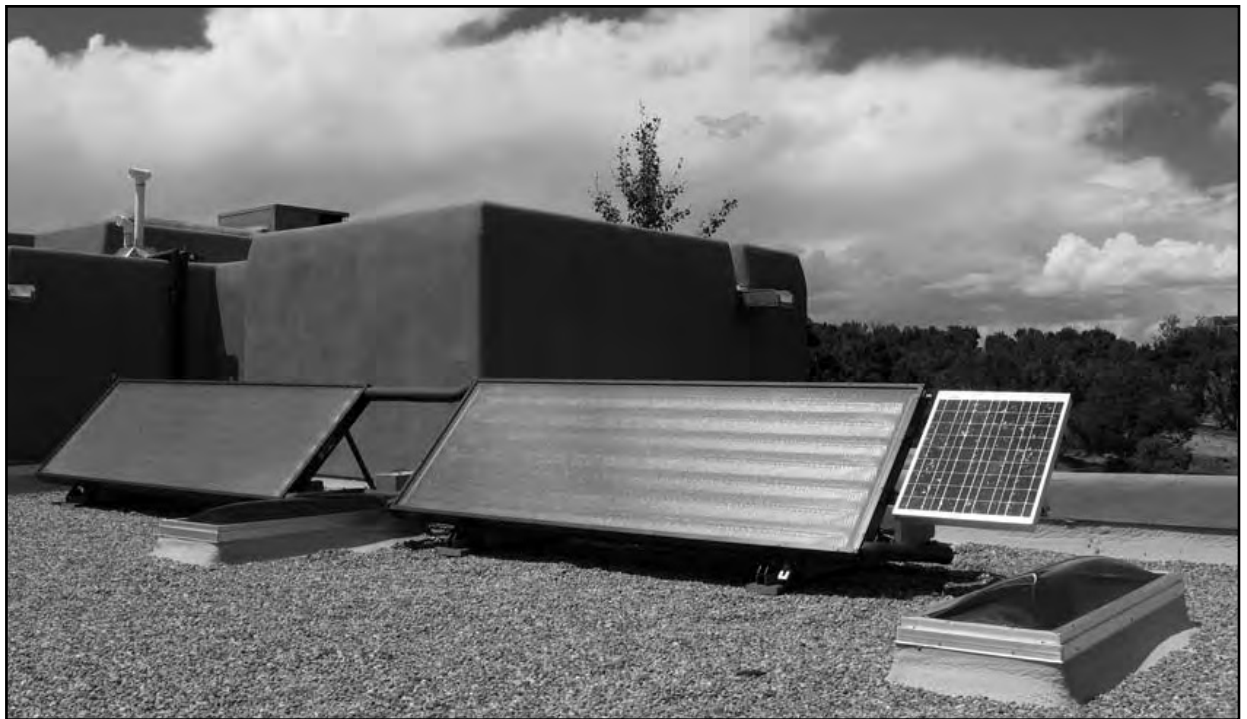
New Mexico has excellent potential for solar water heating (as shown above, on the author's house) and solar PV electricity. Substantial tax credits at the federal and state level make investments in these technologies more attractive. Other large incentives are available for residential solar PV for PNM customers. (Photo by David Van Winkle)
